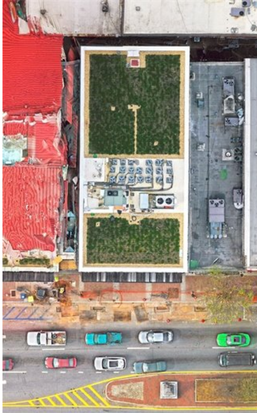
In 2021, the Stormwater Management Program recognized the Green Roof System on top of Target in downtown Athens, designed by Smith Planning Group and grown by James Greenhouses
