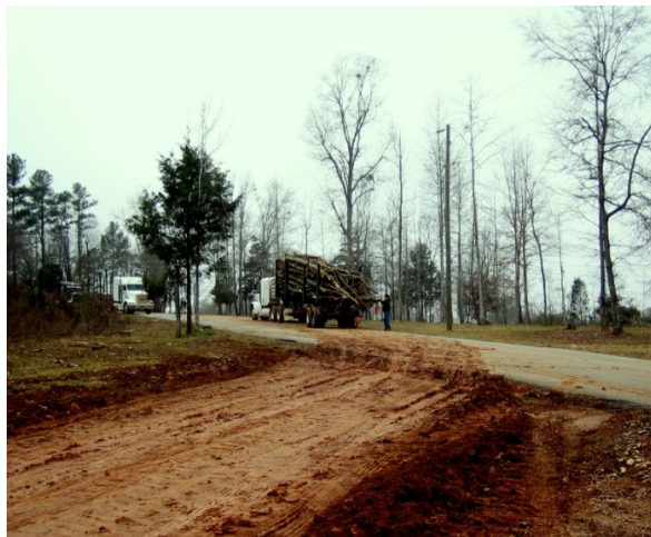
Tracking due to improper site preparation.
