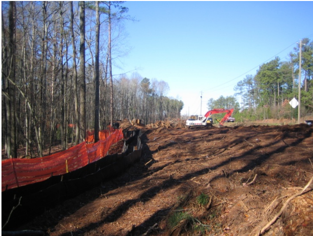
Tree protection fencing and silt fencing properly installed at a timber harvesting site.
